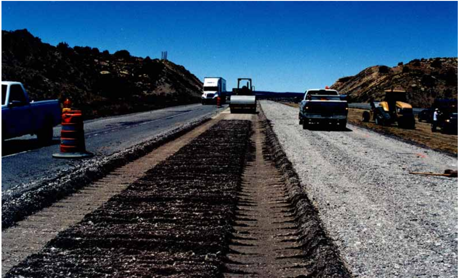
View behind Roto Trimmer showing compaction of the recycled pavement aggregate material in progress following pulverization and treatment with EMC SQUARED Stabilizer solution
